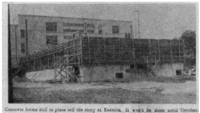
Concrete forms still in place tell the story at Eastern. It won't be done until October.
